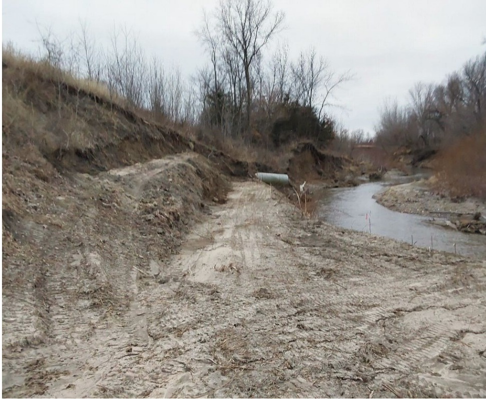
Decatur County Steel Creek project. The beginning stages of stabilizing the stream bank consist of benching the bank for stabilization and the installation of rip rap.
